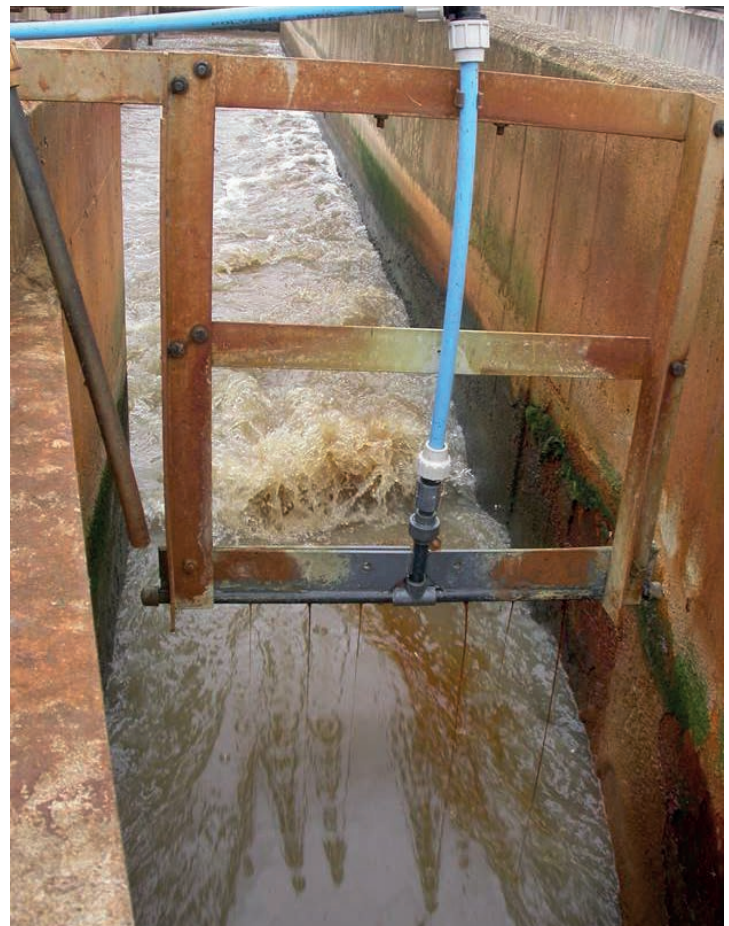
Image of Ferric dosing
